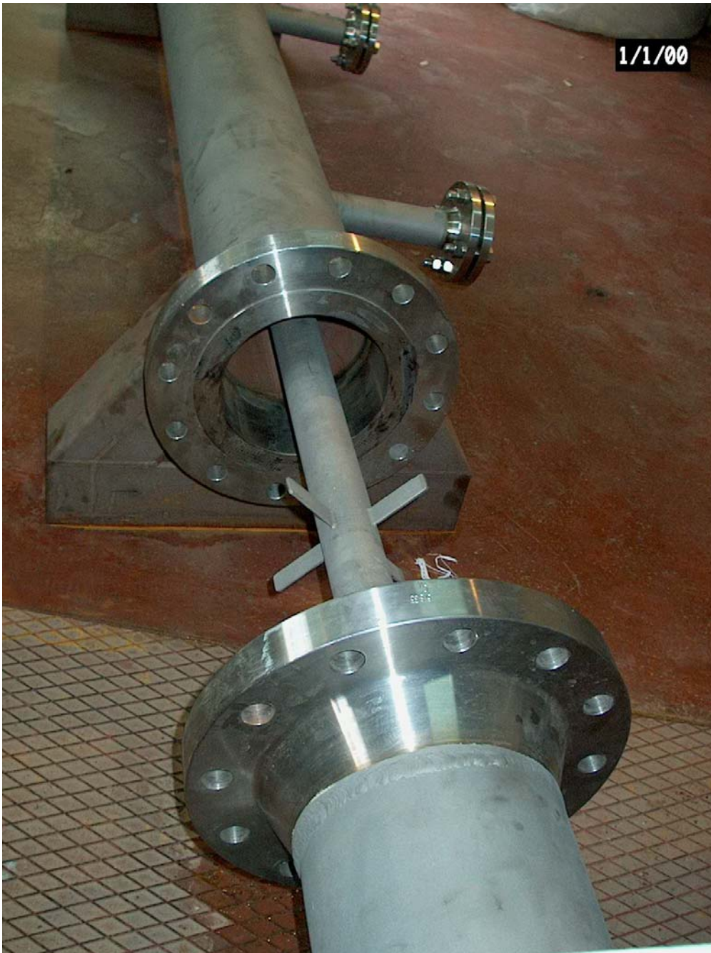
Fig 9.7 Internal water pipe for water injection
